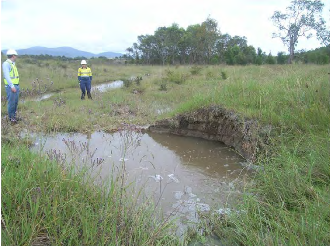
Figure 11. Just upstream of Point S on the map of Gilbert and Sutherland (1997), near the outlet of the sediment dam, photographed in February 2012. The bund has eroded, allowing the creek to flow south of the bund.
